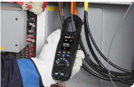
Verify amperage measurements
