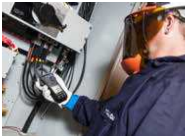
Analyze Power-related Issues
